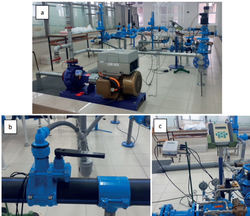
Figure 2. Pressured pipeline system installed at the Hydraulic Laboratory of the Faculty of Civil Engineering, University of Zagreb (a – pump at the inflow section of physical model, b – part of pipeline with nozzle and plate valve to regulate leakage through opening-crack, c – acquisition system controls for dynamic pressure and flow measurement)
