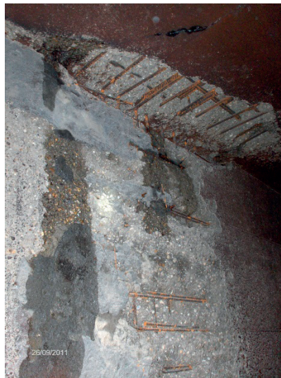
Figure 4. Damage in channels of FES (eroded canal surface with exposed reinforcement steel)
