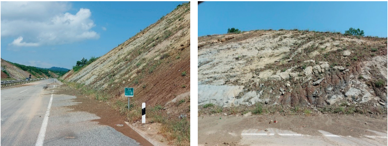
Figure 4. Significant erosion on the slopes between the 2 extreme rainfall events on 29 May 2022
