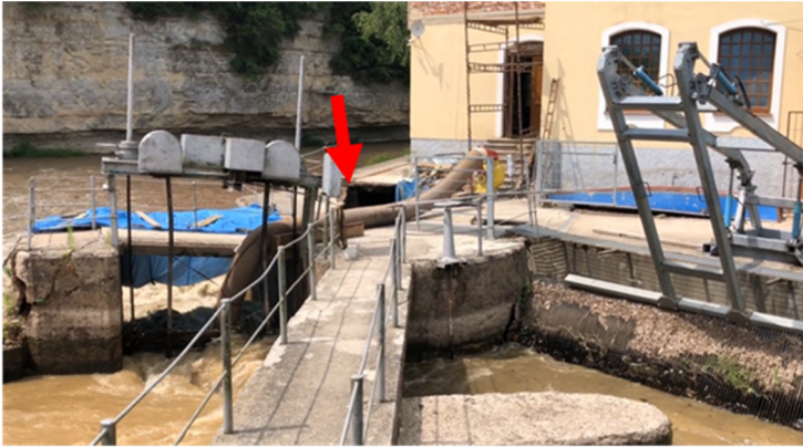
Figure 5. The downstream view at the sluice, the arrow indicates subsidence of the backfill and platform behind the right sluice pier.
