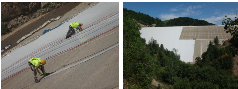
Figure 4. Runcu dam: Heat seaming of overlapping anchor strips and of waterproofing liner to anchor strips
