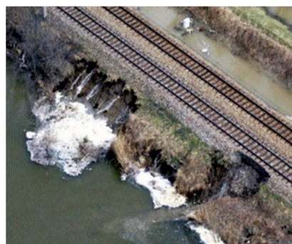
Figure 11. Piping through a railway embankment during an already sinking flood. Train traffic was stopped in 2014 [20].
