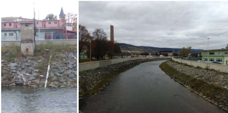
Figure 7. Gauging station on the Topľa River and realized flood protection walls (phase I.) [8]
