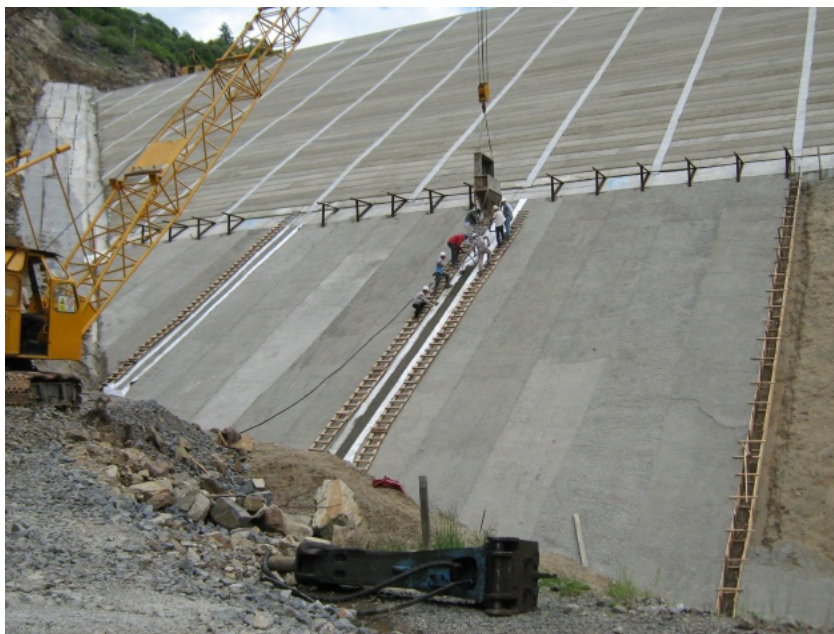
Figure 3. Runcu dam: Anchorage lines in the bottom section are by PVC anchor strips embedded in excavated trenches, in the top section by PVC anchor strips secured to extruded curbs forming the face of the embankment
