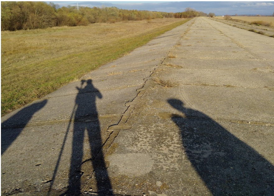
Figure 3. Illustration of the constructed 250 m long solid lateral spillway in the left-side protection dyke
