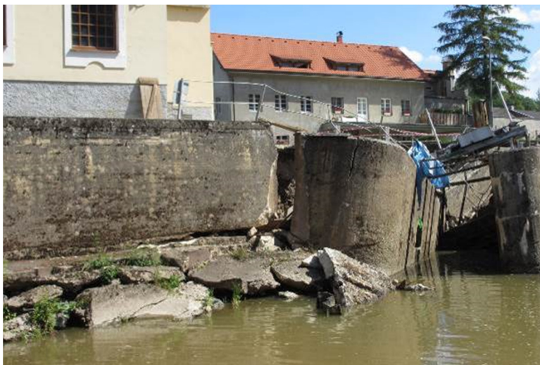
Figure 9. Cracked toe of the right bank wall (upstream view)
