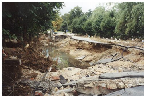
Figure 13. The result of surface erosion of the crest with asphalt pavement during a flood in Czech Republic 2002, [1].
