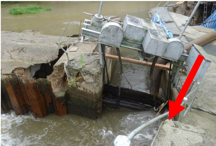
Figure 6. The detailed view at the collapsed right sluice pier with sunk sheet pile.
