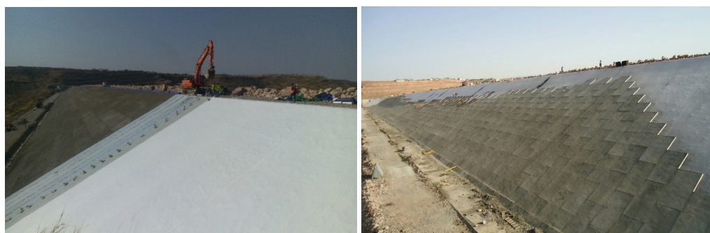
Figure 8. Zarema May Day dam: At left, placement of the decoupling geotextile on the waterproofing geocomposite, at right casting of the unreinforced ballast slabs
