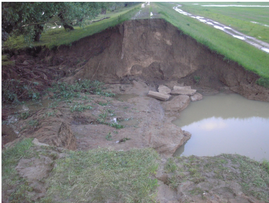
Figure 1. Damaged left side protection dyke on the Ondava River in 2004
