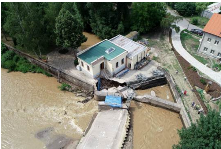
Figure 7. An overall view on the collapsed weir
