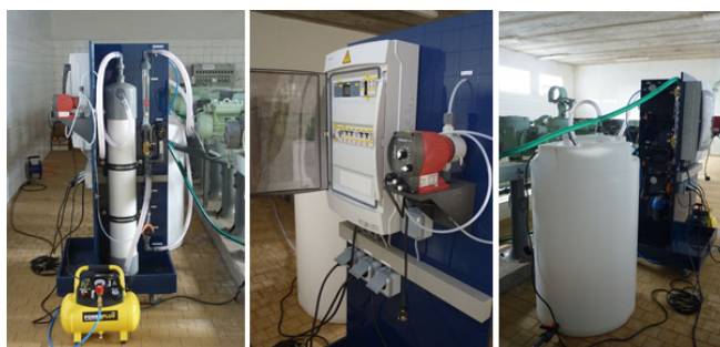
Figure 2. A view of the ultrafiltration device, the membrane module itself, the control system and the treated water storage tank
