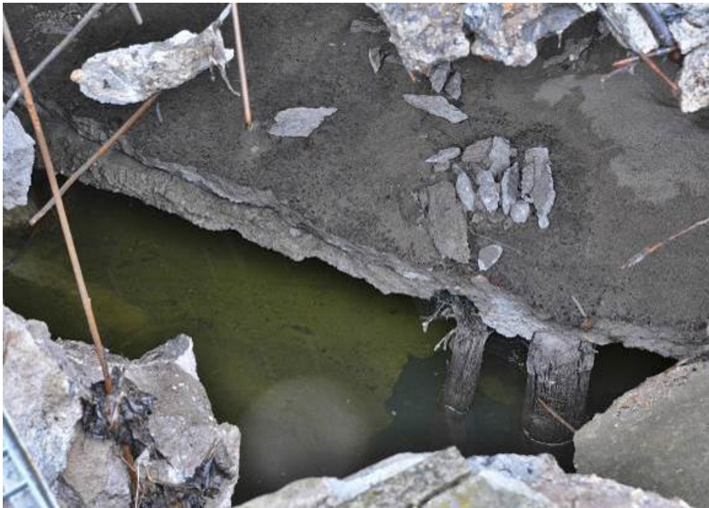
Figure 10. Piles supporting the undermined foundation slab of the HPP inlet
