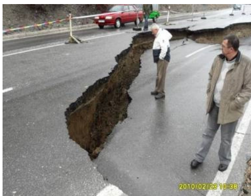
Landslide on the road Bitola – Resen in 2010
