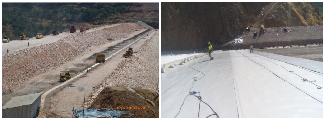
Figure 7. Zarema May Day dam: At left, the sections under (bituminous core) and above (no core) elevation 939. At right, placement and seaming of SIBELON® CNT 3950 geocomposite sheets
