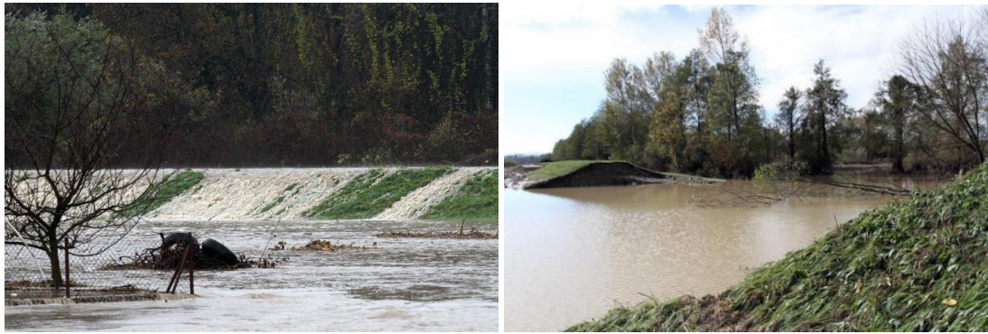
Figure 5. Overtopping and breaching of Otok Virje – Brezje flood protection embankment.
