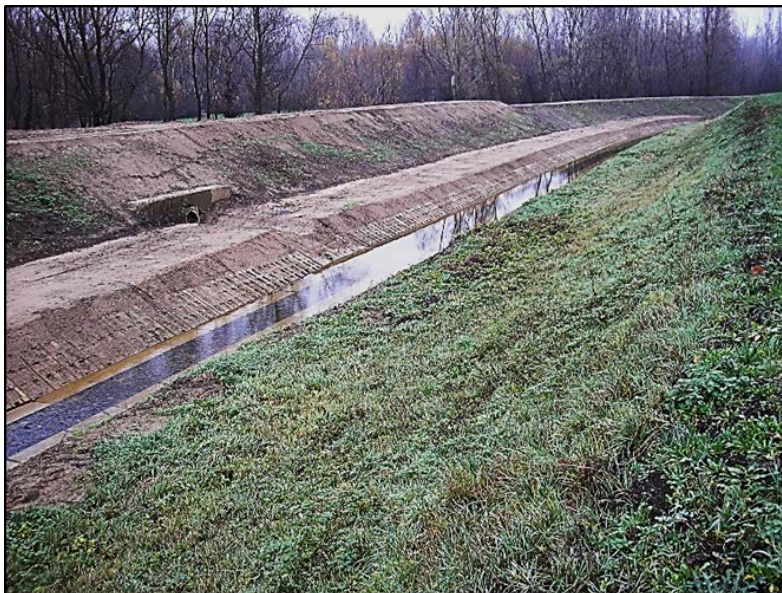
Fig. 6 Adjustment of the left-hand bank of the Borša creek dyke and the spillway, Photo: Tibor Karnay, 2011
