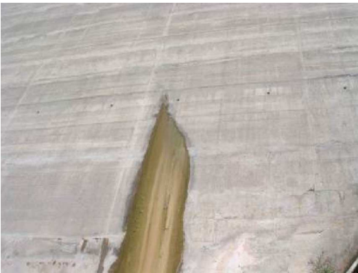
Fig. 5 Rialb Dam (2006), leakage through the crack [photo: Řiha]
