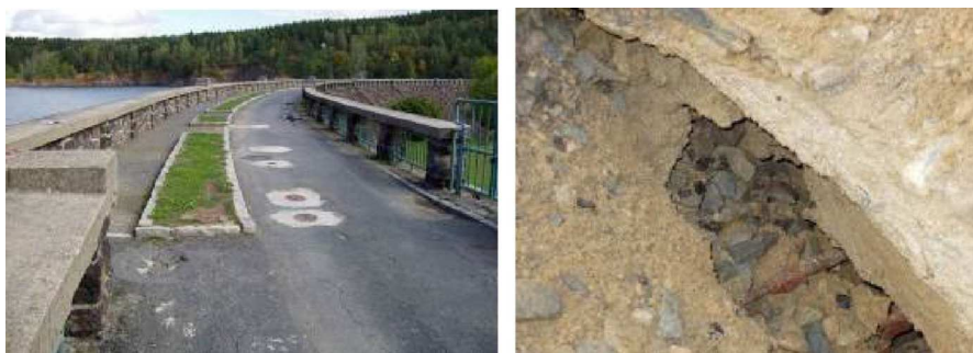
Fig. 9 Mostišť (2004), piping through dam core [photo VD - TBD a.s.]
