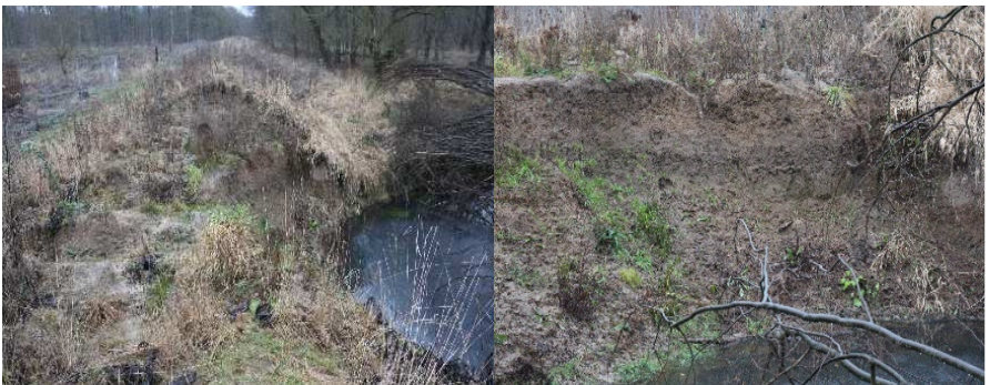
Fig. 3 Typical breach appearance (left) at quasi-homogeneous levees (“old” levees) with distinctive stratification of the levee body (right)
