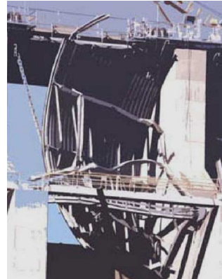
Fig. 6 Folsom dam (1995), gate failure [Vogel, 2014]
