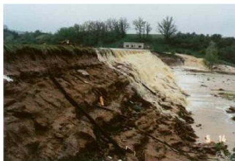
Fig. 8 Pocheň (1997), overtopping and surface erosion [photo: Žatecký 1997]
