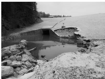
Fig. 3 The scour hole on the left side of the stilling basin prior to refurbishment works
