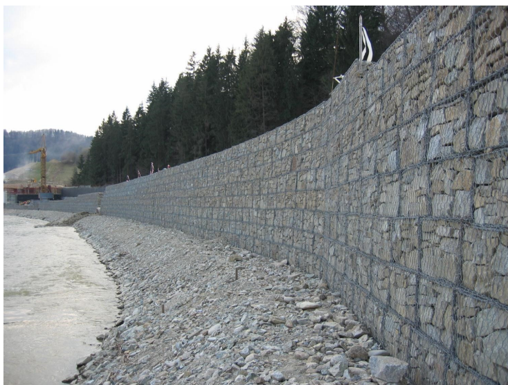
Fig. 4 Gabion river wall at Oravský Podzámok, Slovakia
