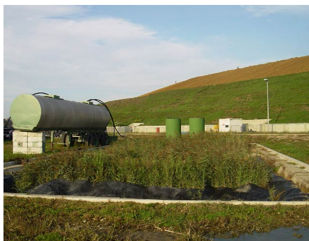
Fig. 5 Constructed wetland Jakuševac (URL_2)
