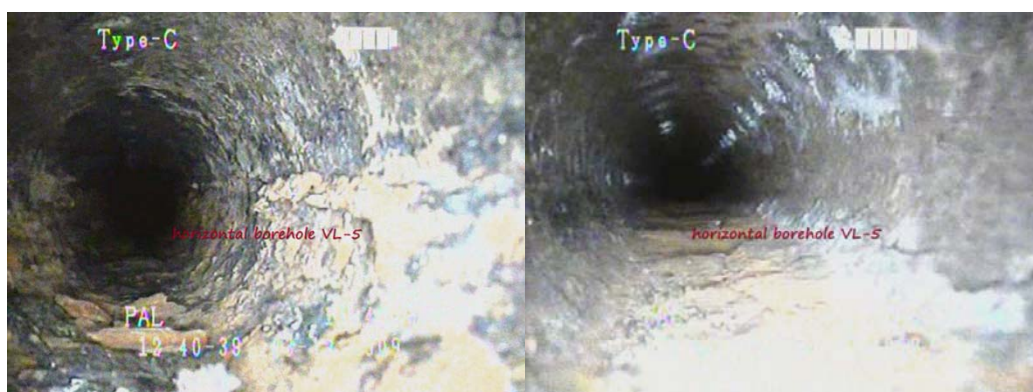
Fig. 6 State of the HDB casting after 38 years in operation at the camera inspection
