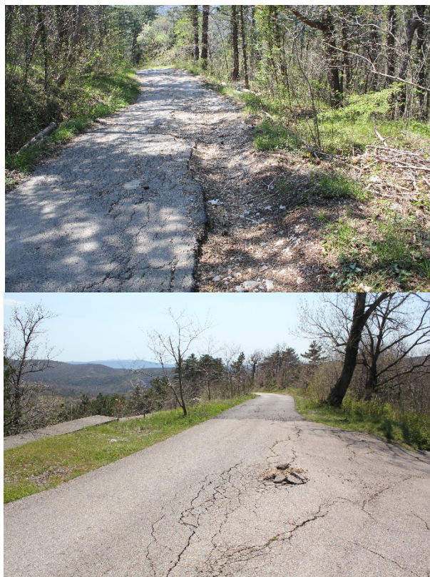
Fig. 8: Result of erosion processes and soil instability on the road between sub-catchments Slani Potok and Mala Dubračina
