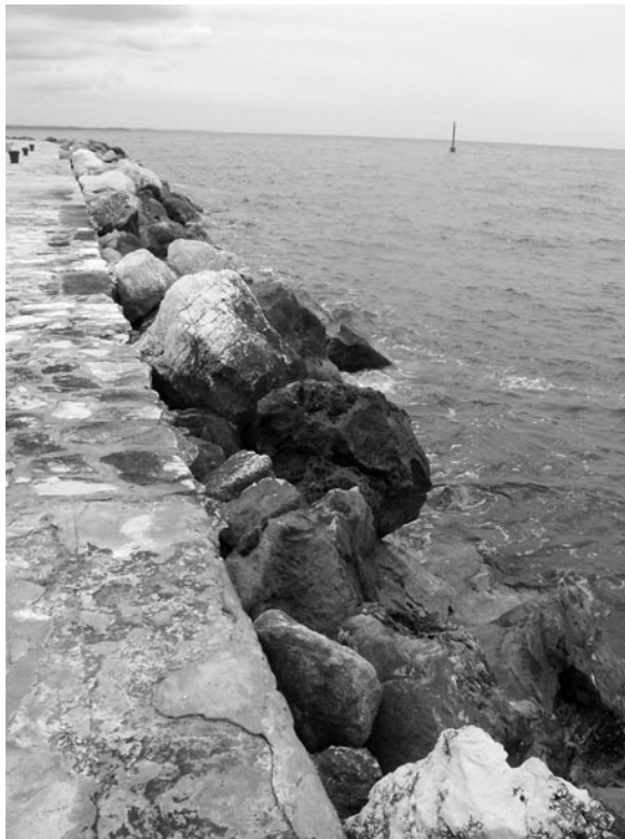
Fig. 6. A detail of the damage on the breakwater's slope in Novigrad
