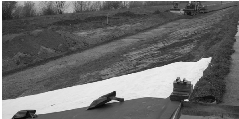
Fig. 2. Realization of the sealing of the upstream slope of flood dyke (Photo: Sabo J.)
