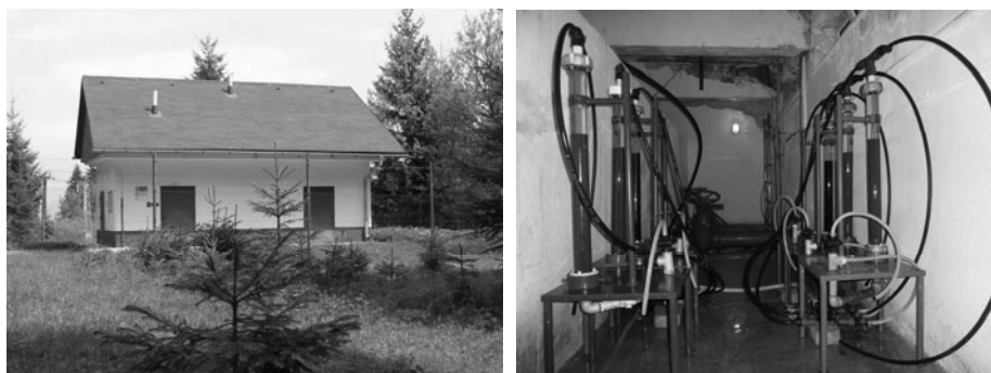
Fig.1. Dúbrava chlorination plant and model filtration columns
