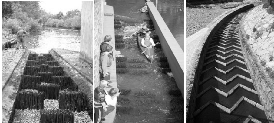
Fig. 2. Detail of the brush elements in the slip-way and slip-way with retarding elements
