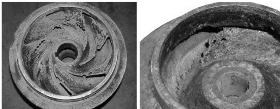
Fig. 2. Typical cavitation pitting in impeller [5, 6]
