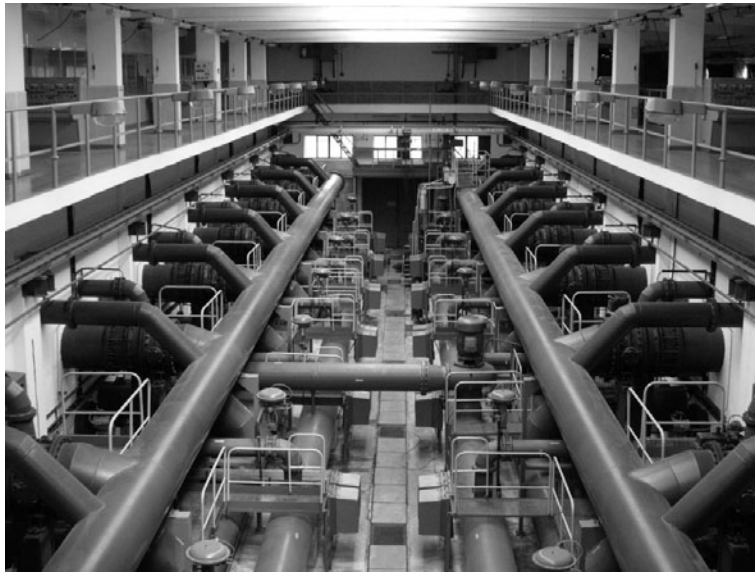
Fig. 3. Technical systems at the surface water intake in Straszyn
