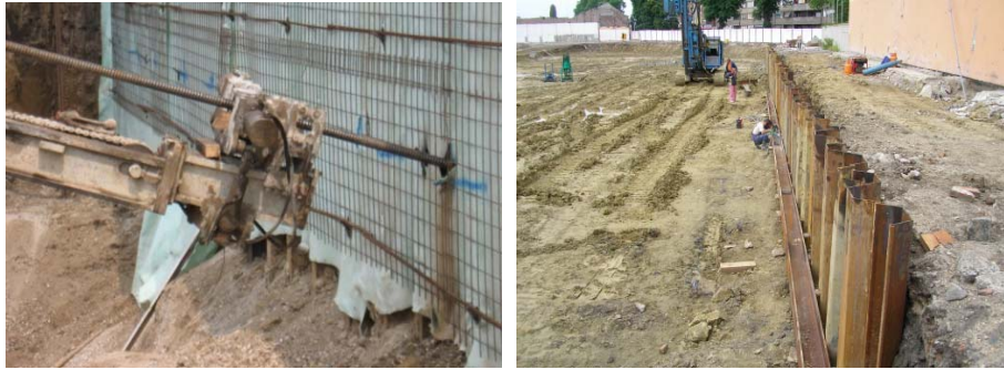
Fig. 4. Construction of steel sheet piling supporting by anchoring (trade center Interspar in Osijek): (left) drilling of anchor layer by special machine, (right) installation of main beam
