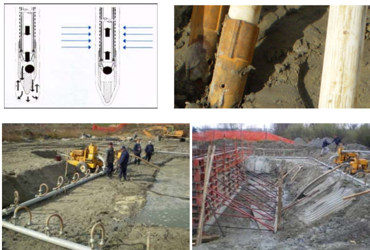
Fig. 8. Application of wellpoint in the area of old bed of the Drava near Osijek: (up) head of the pipe filter (PVC), (down) parts of wellpoint machine on the building site of sewer pumping station Bilje
