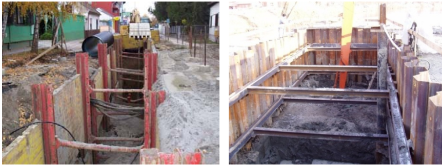
Fig. 1. Krings Verbau formwork system and steel planks driving make main sewer excavation protection
