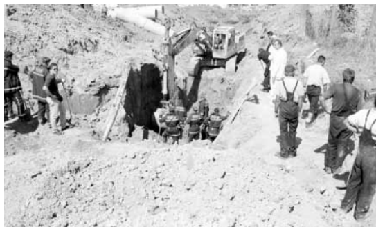
Fig. 2. After caving situation on the building site of sewer collector when two workers of the firm Vodovod tragically died (Vjesnik, 01.09.2001.)
