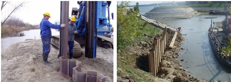
Fig. 3. Construction of building pit protection at bridge pier in the bed of the river Bosut in Vinkovci: phase of dike construction in the bed and driving of steel planks (left), example of permanent support at quay construction in Vukovar port for putting to shore of small vessels (right)
