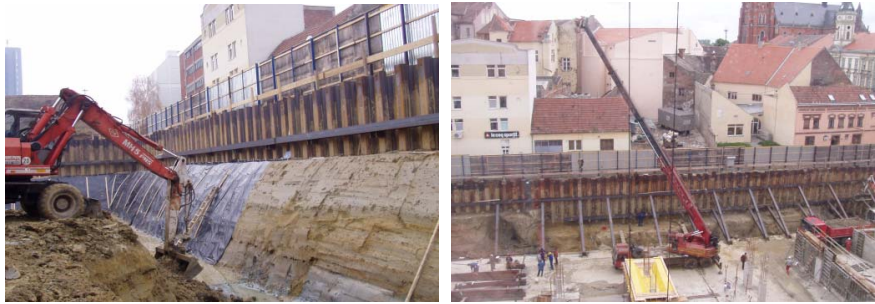
Fig. 5. Building pit protection by steel sheet piling of Esseker center in Osijek: (left) ground excavation in protected building pit, (right) supporting of steel sheet piling by diagonal bracing
