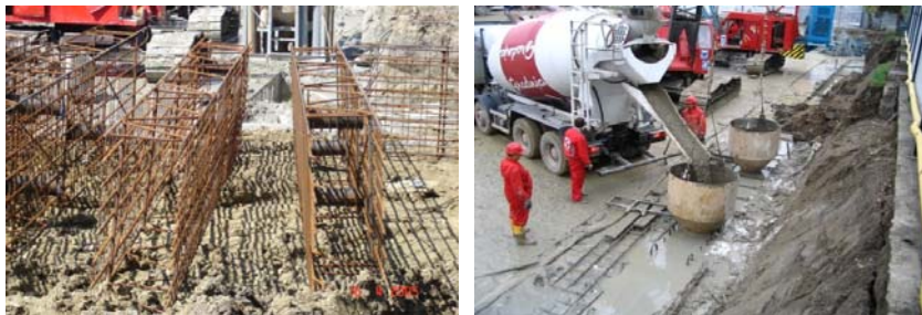
Fig. 7. Eurodom Osijek: (left) reinforcing cage for building of diaphragm wall, (right) concreting of diaphragm by contractor procedure
