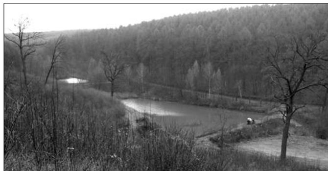
Fig. 4. Situation of the area of interest and view to upstream face of the earth dike of water reservoir Koberice, which is called Bezednik III (the name means without the bottom)
