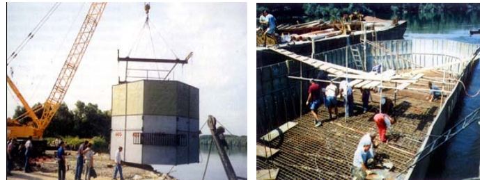
Fig. 11. Steel formwork application for making the works possible on dry when constructing the bridge prier in the river bed (Drava near Belišće)
