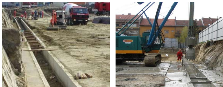
Fig. 6. Construction of diaphragm wall on multipurpose object Eurodom in Osijek: (left) construction of introduction channel, (right) trench excavation for diaphragm by special equipment
