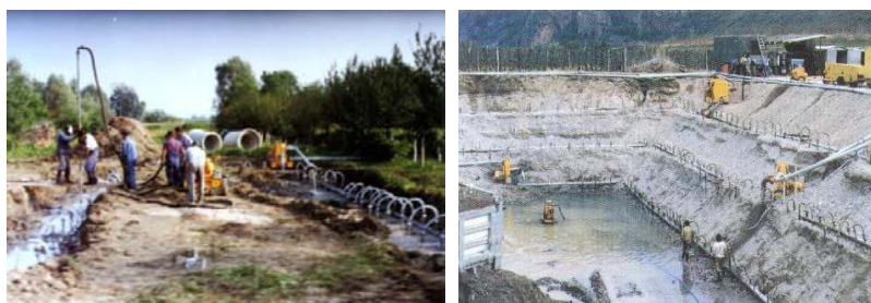
Fig. 9. Application of wellpoint system on one level near Donji Miholjac (left), decreasing of underground water level on bigger depths on more levels (right)
