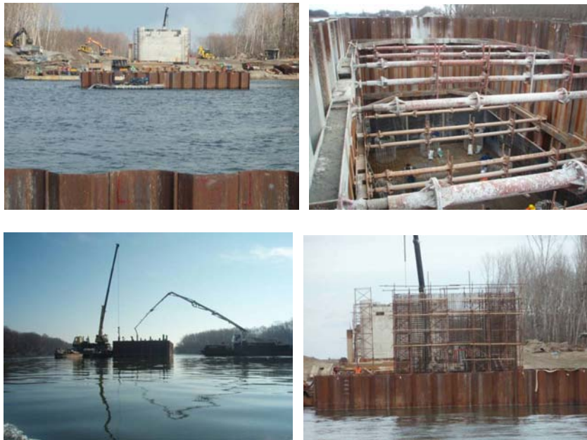
Fig. 10. Building pit in the river bed: it shows the protection by closed series of planks reciprocally braced, pumping of seepage water and some building works
