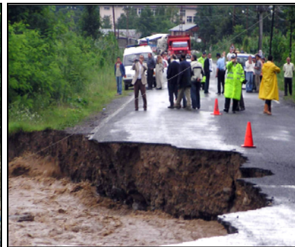
Fig. 5. Caykara road (after the flood)[6]
