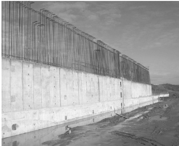
Figure 10 Construction of west part of front wall at its half high (November 2003)
