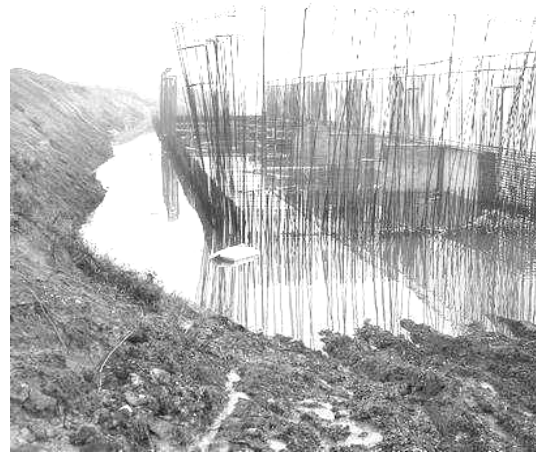
Figure 7 Flood, after front wall was erected (October 2003)
