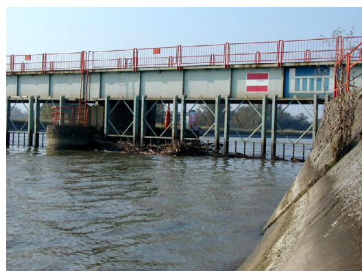
Fig. 7 Intake structure of the inlet channel – clogging of coarse rack
