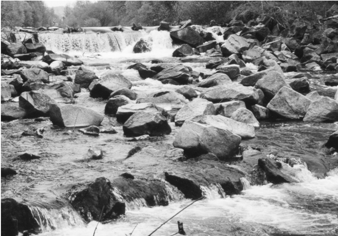
Figure 3 Example of a fish migration barrier due to subsidence of a ramp after decades because of insufficient filter construction
